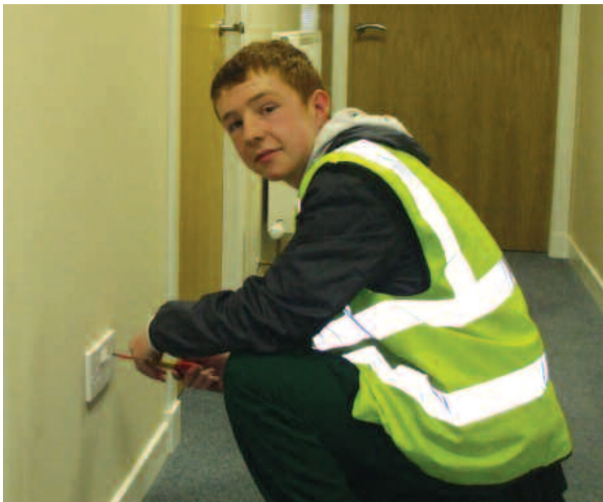
Above, we see Gary checking out an electrical socket.
